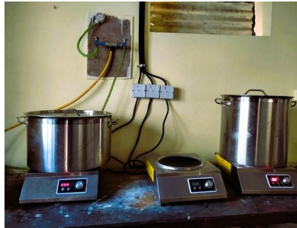
Figure 15: Electric induction hotplates in the kitchen
