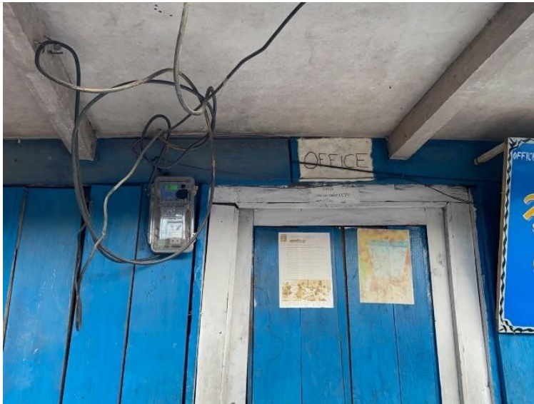
Figure 7: "Office" power connection, Grey school building, Nepal
