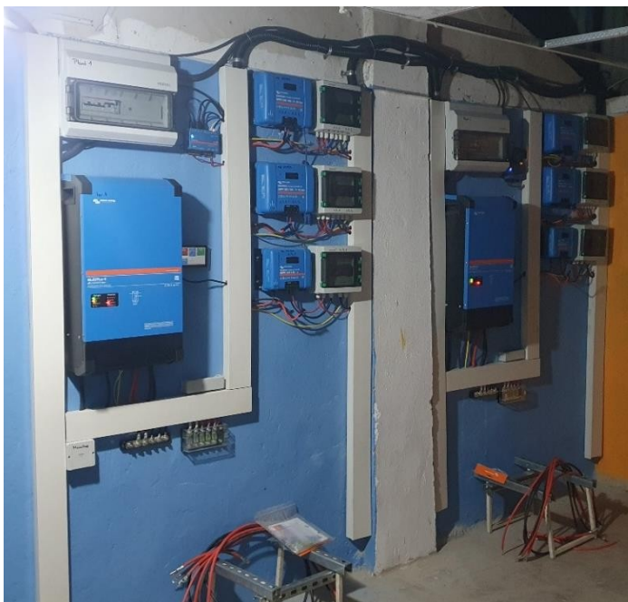
Figure 12: Fully assembled system 1 and 2
